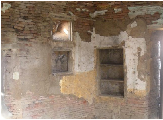
Figure 12: Damaged traditional masonry and mud plaster
