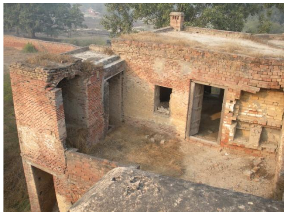
Figure 11: Staircase part detached from main building
