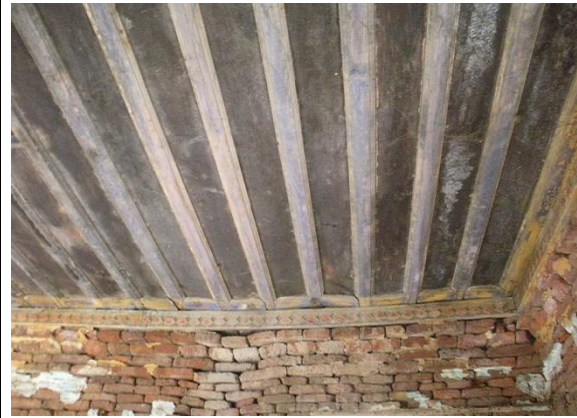
Figure 13: Damaged traditional khatambandi ceiling
